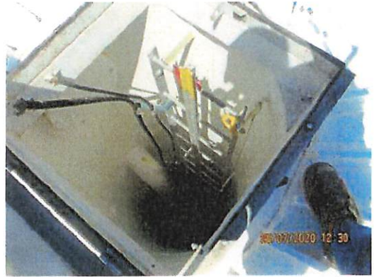
Dry riser hatchway open for roof access
