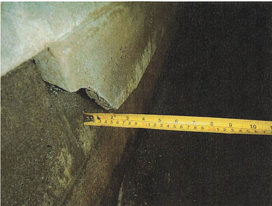
Photo 26. Photo illustrating 2" shift in addition foundation wall
