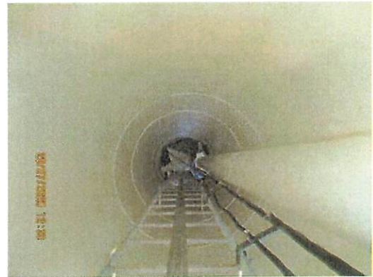
View straight down the dry riser and ladder
