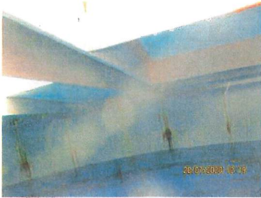
Typical internal wall view of coating failures
