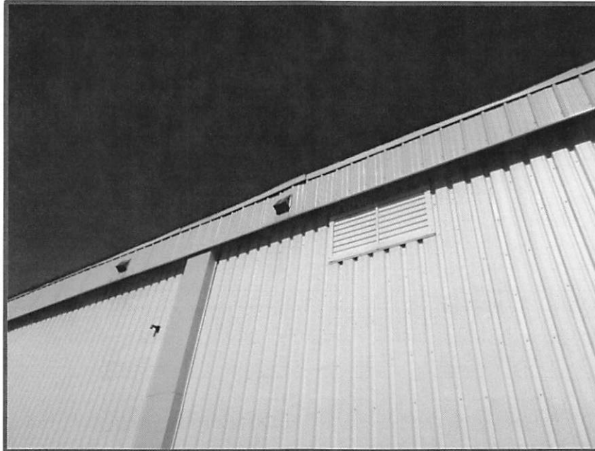
Photo 9: Loose Fascia Siding
