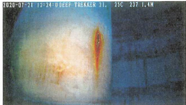
Coating failure on dry riser
