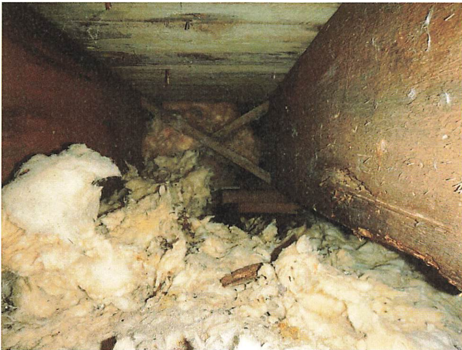
Photo 20. Damp batt insulation found in crawlspace under NW bathroom
