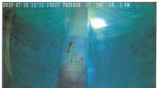
Coating failure at the water level fluctuation zone
