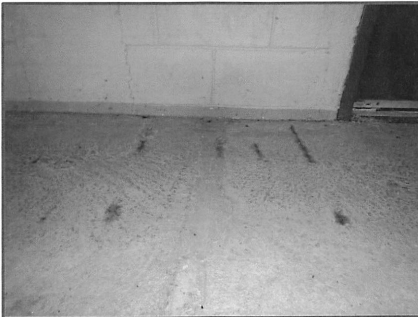
Photo 28: Rebar Staining in Bleachers Concrete
