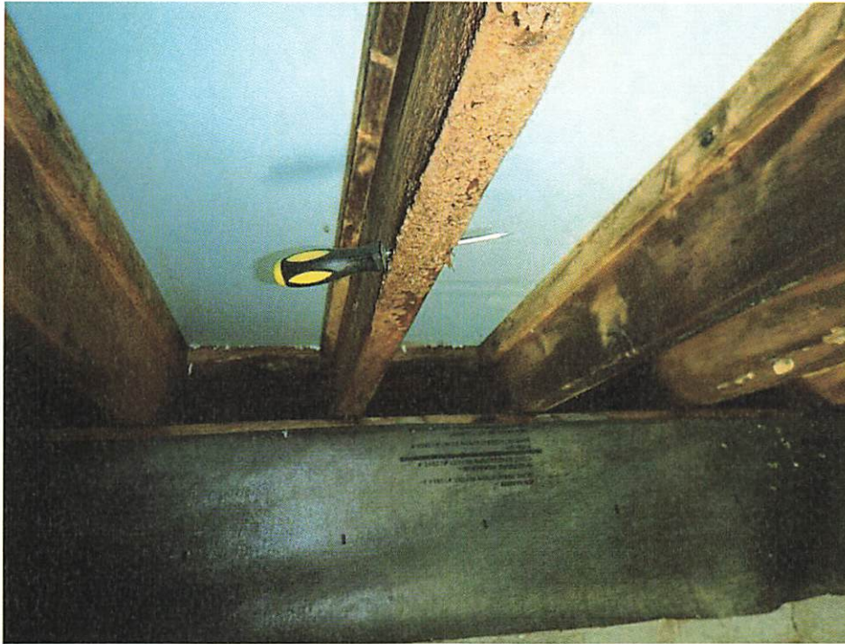
Photo 27. Photo illustrating extent of rot in addition floor joists
