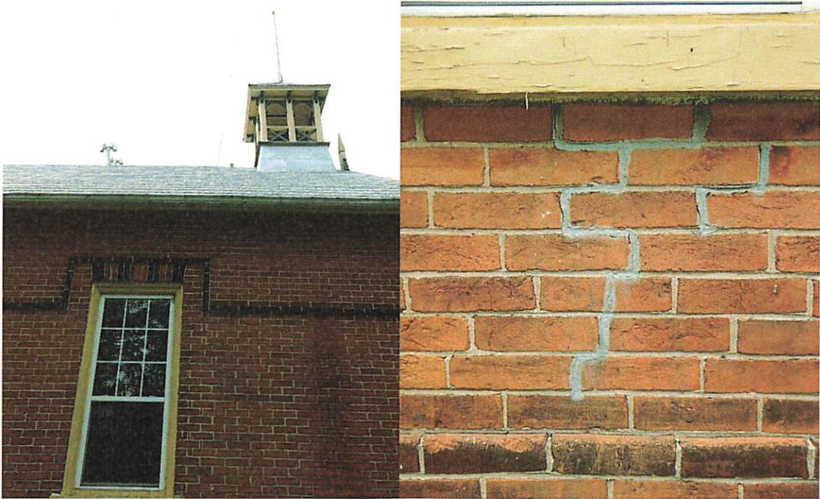
Photo 11. Localized step cracking in brick wall (several locations have been previously repaired)
