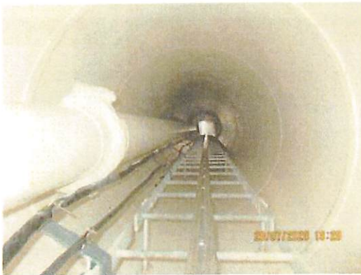
View directly up dry riser; roof hatch secured
