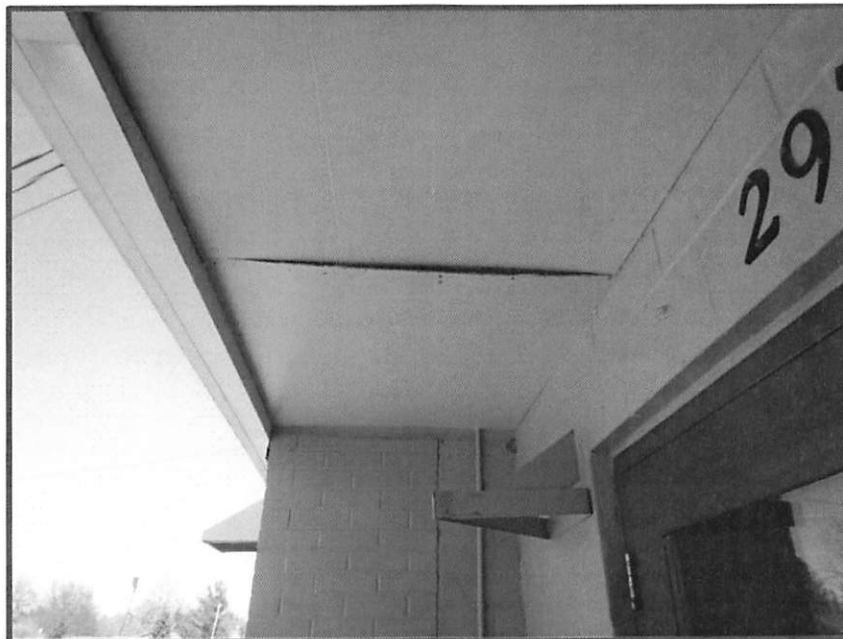
Photo 16: Loose Soffit at Entrance
