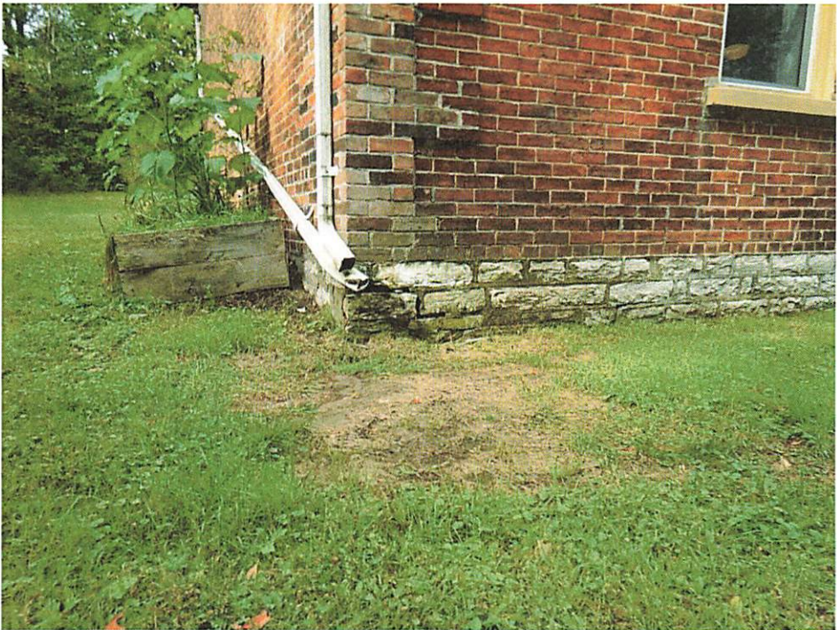
Photo 10. Water pooling and mortar loss at SE building corner
