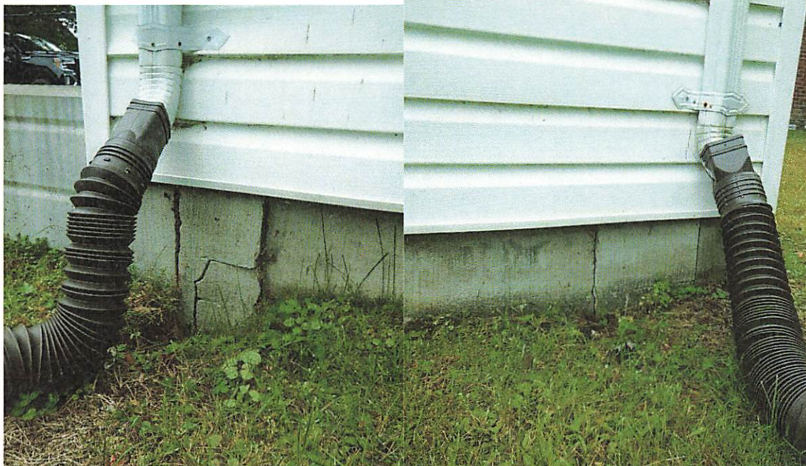
Photo 6a. Localized cracking in NW foundation
