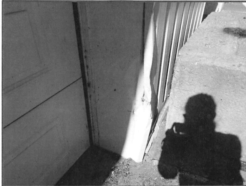
Photo 15: Damaged Siding at East Elevation
