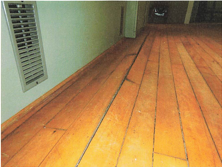
Photo 16. One location of heaved floorboards
