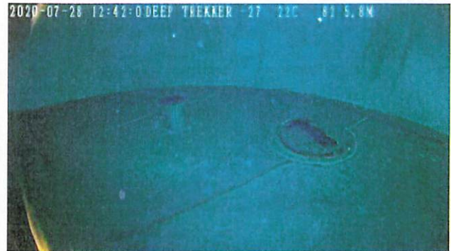
Inlet-outlet pipe, hatch cover, thin sediment layer
