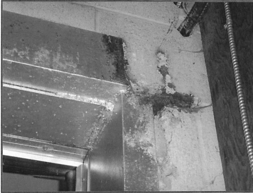
Photo 27: Damage at Zamboni Door
