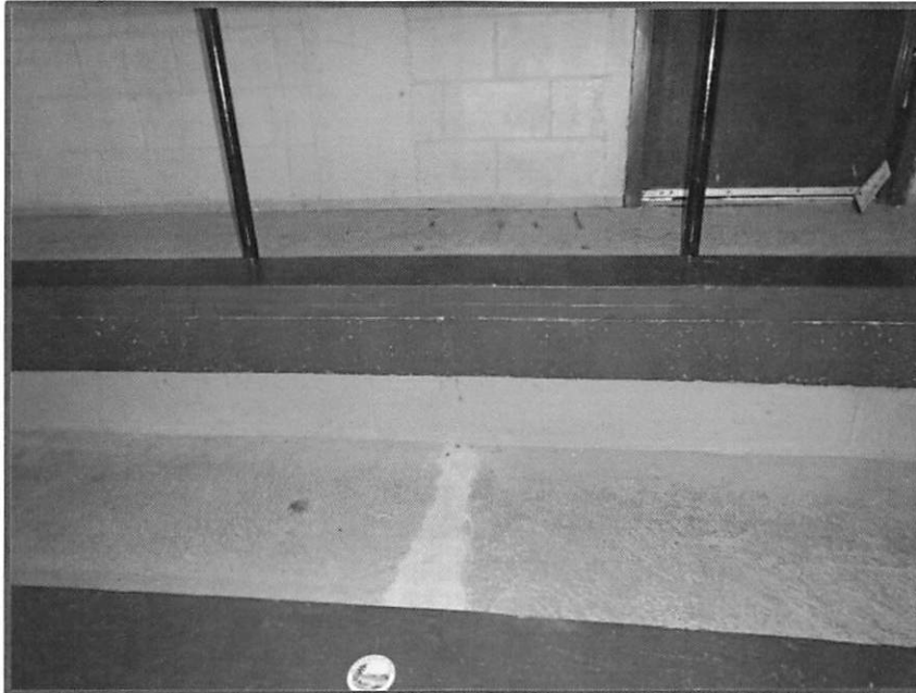
Photo 29: Previous Patches in Concrete Bleachers
