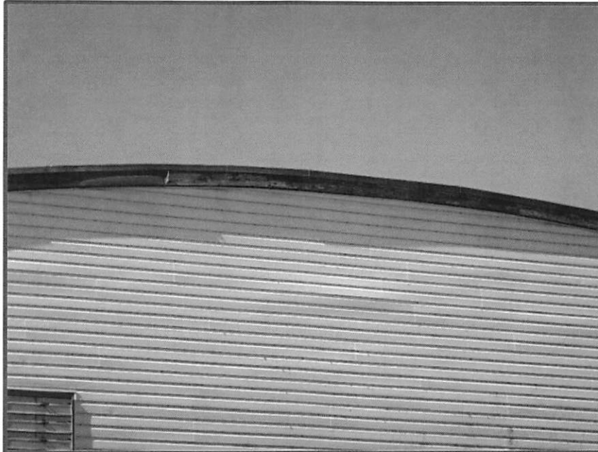
Photo 11: Missing Fascia on East Elevation
