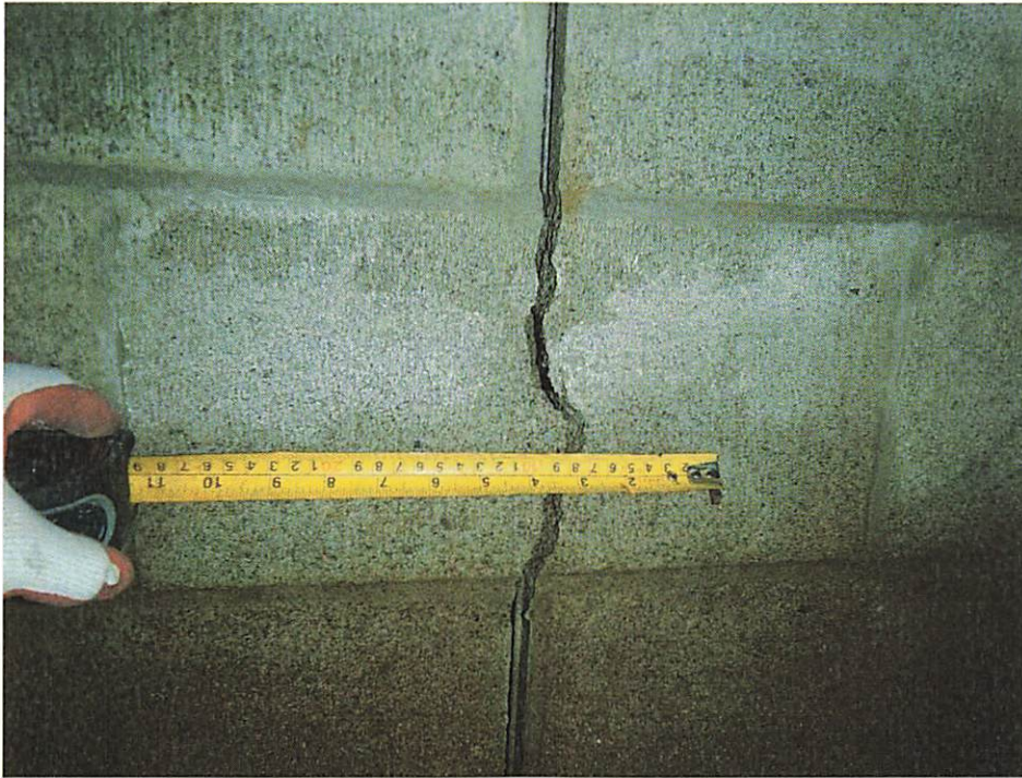
Photo 25. Wide crack in addition foundation wall
