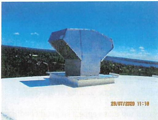
Roof top vent assembly in good condition
