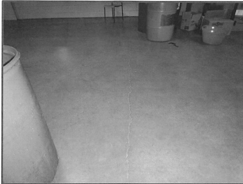
Photo 33: Crack in Concrete Floor on Second Storey Viewing Area
