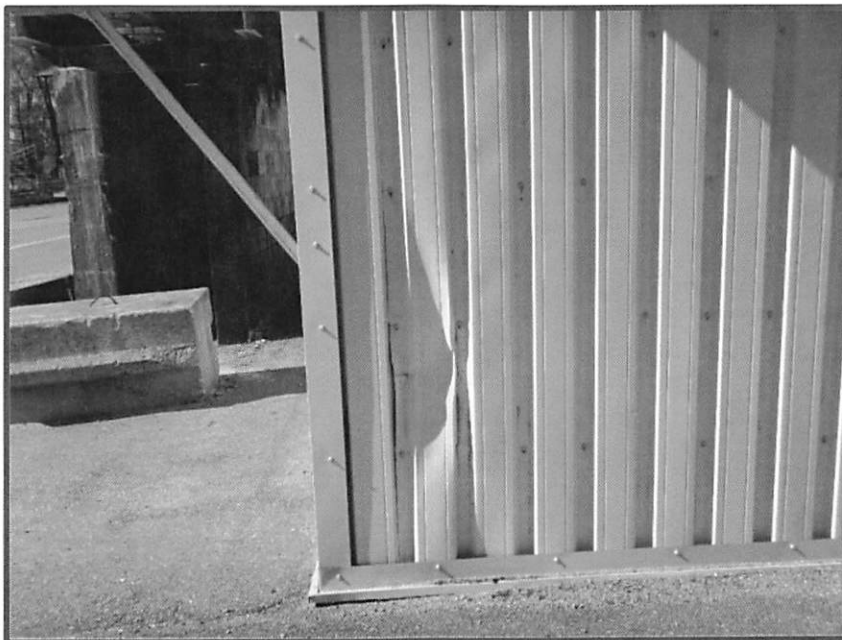
Photo 12: Damaged Siding at Southeast Corner
