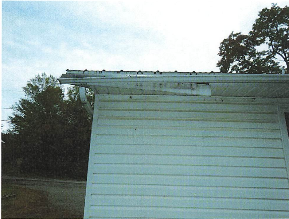
Photo 7. Damaged soffit in addition
