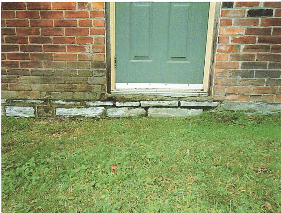
Photo 8. Mortar loss in exterior stacked stone foundation
