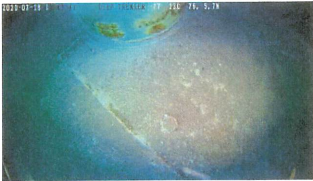
Coating loss at dry riser bottom, thin layer of sediment
